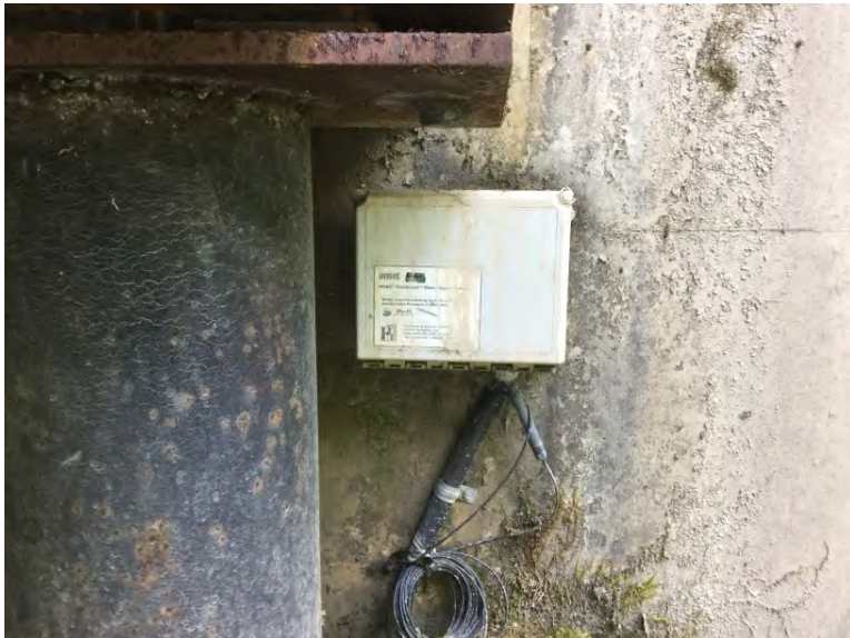
Water level monitoring system
