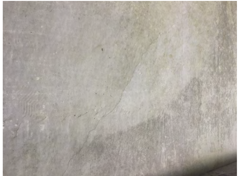
Hairline cracks noted on girders
