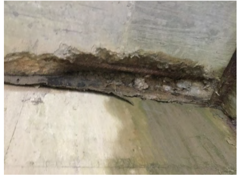
Damage noted to left bank panel
